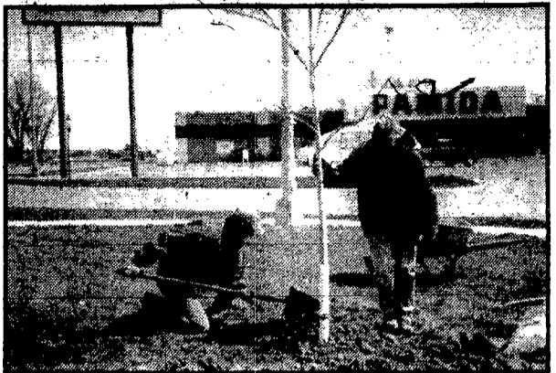
Mike Lutt and Jo Anne Hardisty of Country Nursery plant the last of 40 trees on Monday. This tree was planted near the intersection of Seventh and Dearborn Streets. The tree planting was a result of the Highway 35 Widening project.
